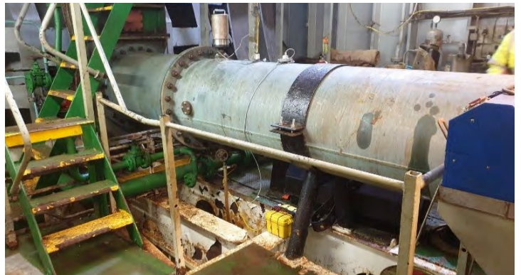
Sensor on pipe
